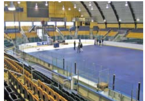
Installation is quick, clean and simple. An average ice arena can be completed in 1-2 hours using 8-10 workers.
